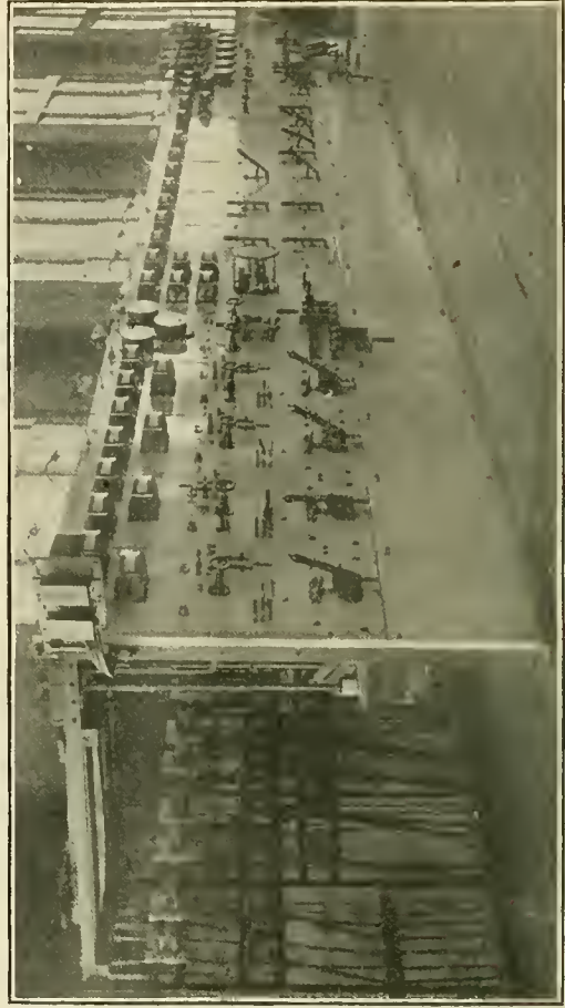
VIEW OF MAIN SWITCHBOARD (B) FOR THE SHOP DISTRIBUTION CIRCUITS. GENERAL ELECTRIC CO.
